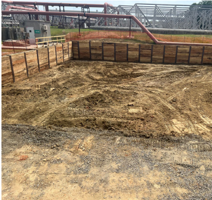
McAlpine Creek Wastewater Mngt Facility WAS Equalization, Blending & Odor Control, Pineville
