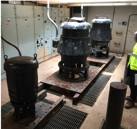
Emergency Generators, DC Water and Sewer
