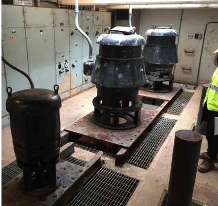
Emergency Generators, DC Water and Sewer
